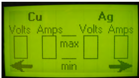
Controller not in Operation
