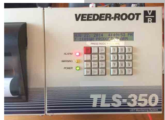
Figure 9.1: Monitoring console in alarm
