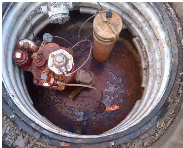
Figure 10.10: Tank top sump with product
