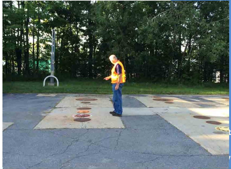
Figure 18.2: Class C operators need to be aware of the basic system components. Class A or B operators should explain the onsite equipment during training.
