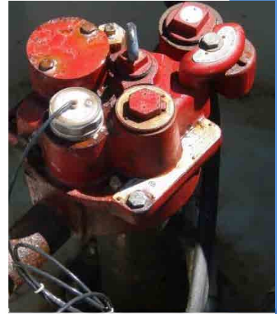
Figure 10.7: Electronic line leak detector on a submersible pump (EPA)
