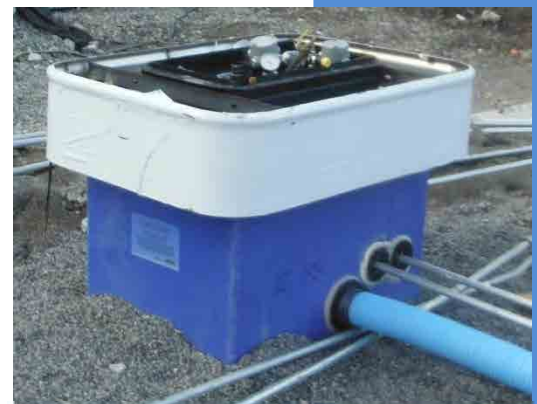
Figure 12.9: UDC with a steel island before burial, showing underground piping and conduit connections.
