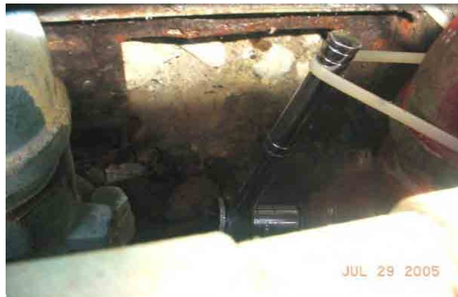
Figure 12.12: Shear valve held open with a socket wrench and zip tie. This, like the shear valve in the previous figure, is a major fire and environmental hazard, and would fail a DEC inspection.
