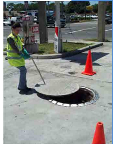
Figure 2.1: Operator opening a tank top sump. Class A and B operators are responsible for tank maintenance and monitoring
