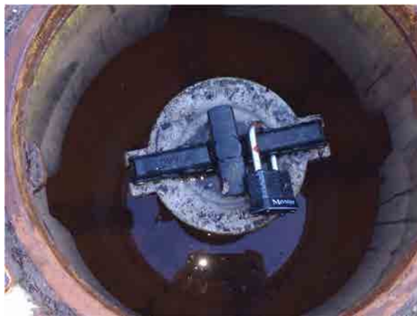
Figure 13.3 Dirty spill bucket in need of cleaning
