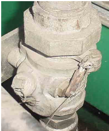
Figure 12.11: Retrofitted shear valve. This defeats the safety purpose of the valve and would fail a DEC inspection.
