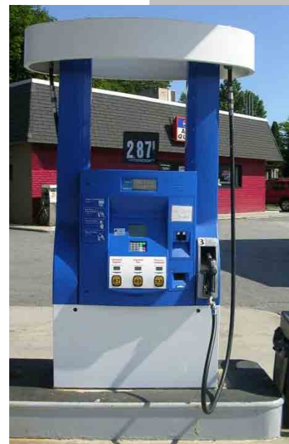
Figure 12.3: Typical retail dispenser
