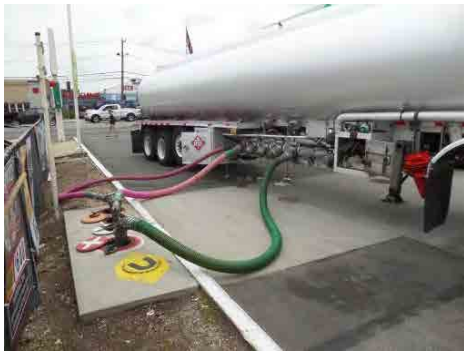
Figure 13.1: Fill hose connected to fill port inside a spill bucket
