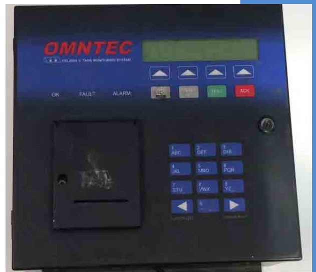
Figure 8.1: ATG system console (example of one make/model)
