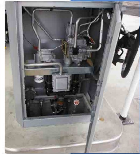
Figure 12.6: Pressurized system dispenser
