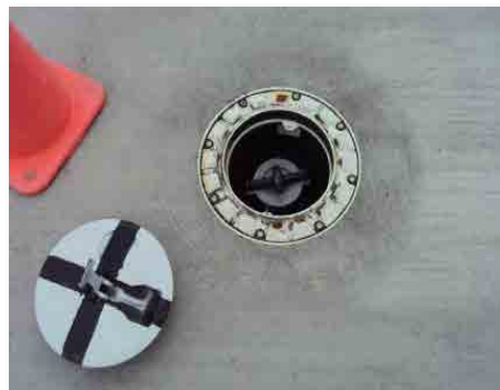
Figure 13.2: Fill port inside spill bucket
