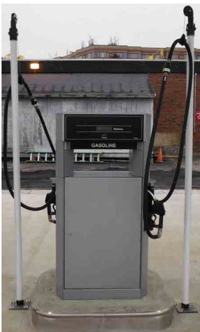
Figure 12.1: Typical fleet dispenser
