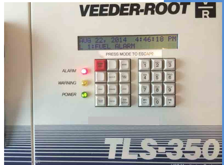
Figure 10.12: Electronic monitoring console in alarm
